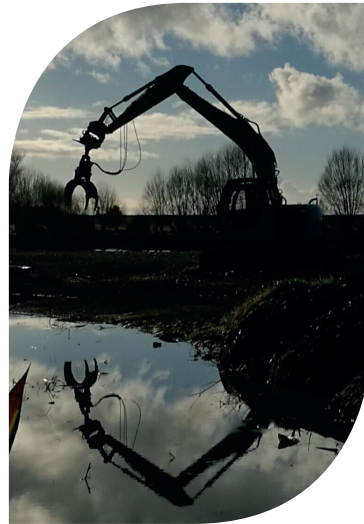
Digger working in late June - all the Willows have gone waiting for low growing flaxes and natives. Some of the flaxes of the Rene Orchiston Collection of 61 cultivars will be planted here. Residents of Kuku Street are very involved with this planting.
